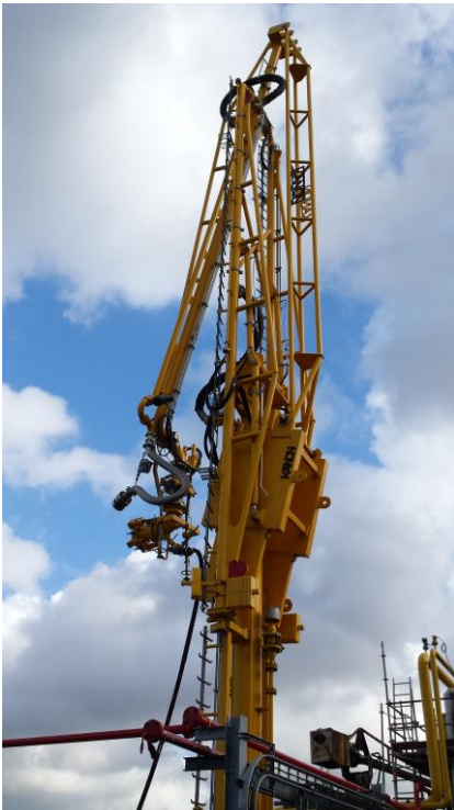
Figure 7. LPG retractile transfer arm at the ATPC facility in Antwerp.
