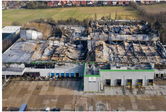
Figure 4. Ocado's fire aftermath, taken from [14]
